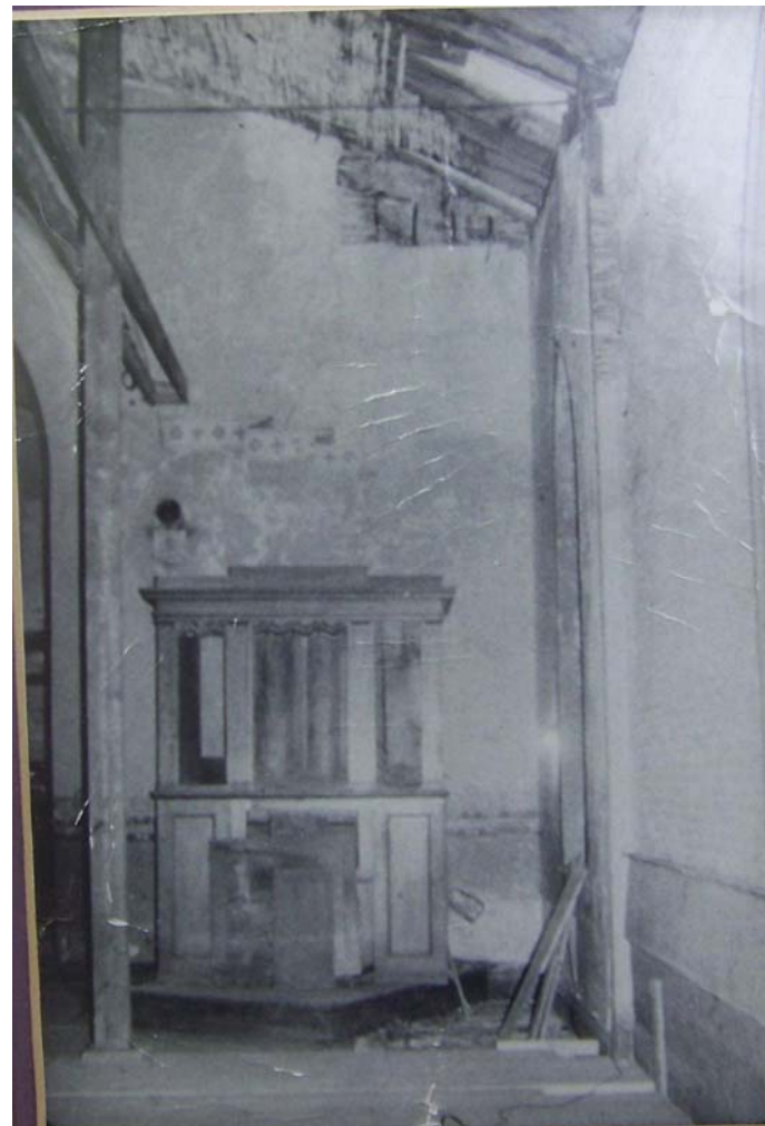
↓ West Nave Wall Showing Issues with Plaster and Roof
